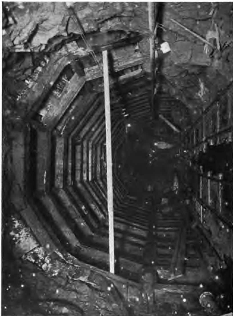
PLATE 87. —Rondout Siphon. Five-piece Arch Timbering in Heavy Limestone South of Shaft 3. This timbering supported longitudinal steel I-beams which were concreted in with arch. Timbering was removed in advance of concrete, leaving I-beams to support roof in stretches of about 15 feet.
